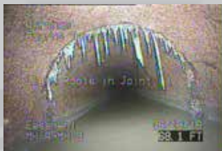
Roots at Joints
